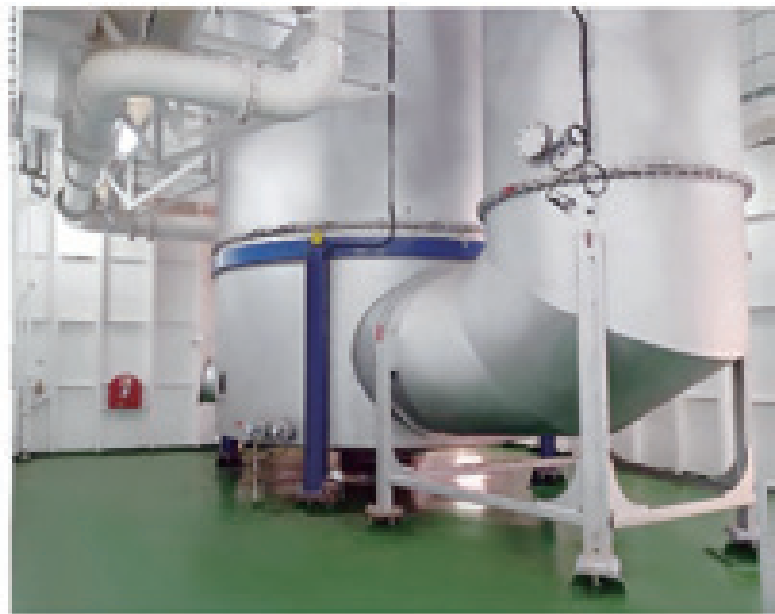
▲ SOx Scrubber system
